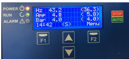
Fig 2.1 Controls/display (1 per pump motor)
