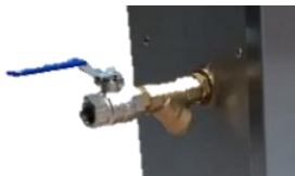
Fig 2.2 Mains water inlet isolation valve & strainer
